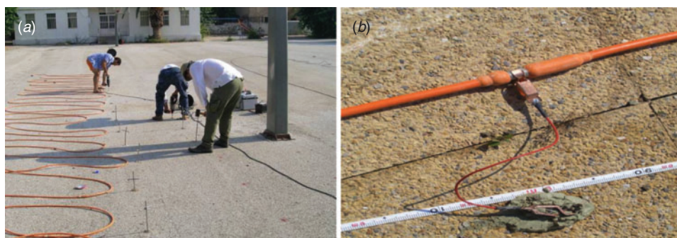
Fig. 2. (a) Field procedure at the area of Turkish School in Rethymno where a pneumatic drill was used to open small holes in order to insert metal stake electrodes in the ground. (b) Bentonite contact electrodes used in the Heraklion investigation.
